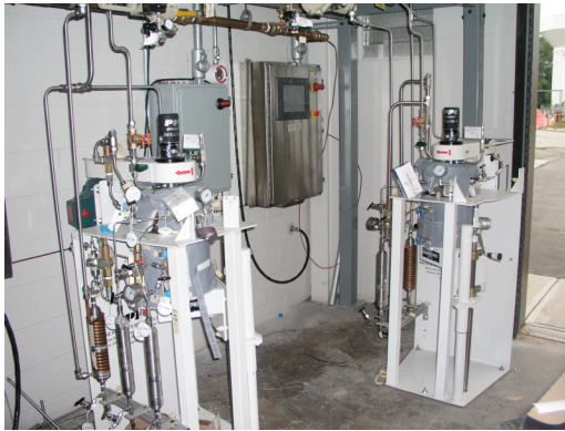
F-T Reactors installed in Alternative Fuel Laboratory
